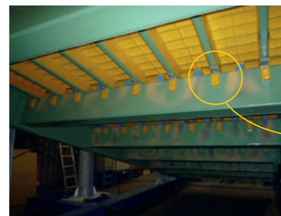
PU rivet protection inside the Screening Machine as wear protection
