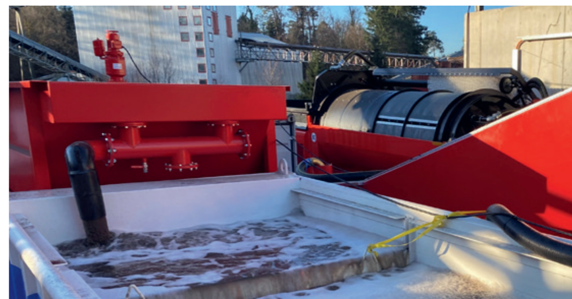
View from above the Lamella Separator
