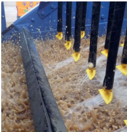
Partial spraying system on the Screening Machine
